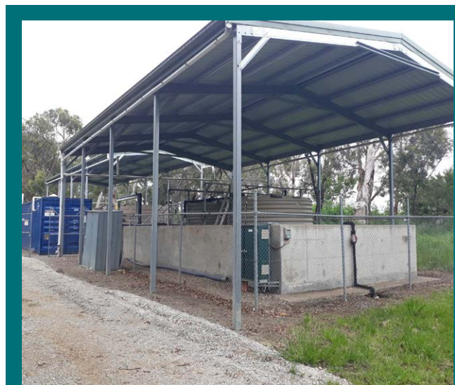
Coldstream leachate plant – the plant processes leachate liquid collected from the landfill for disposal into the sewer system. This is important to ensure that the liquid does not contaminate local groundwater and the surrounding environment.
