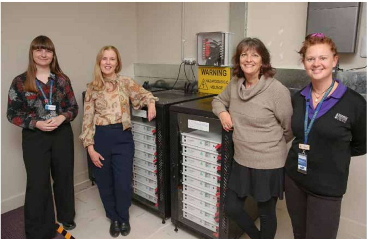
108 kWh battery at the Healesville Library
