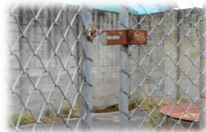
Water mains enclosure
